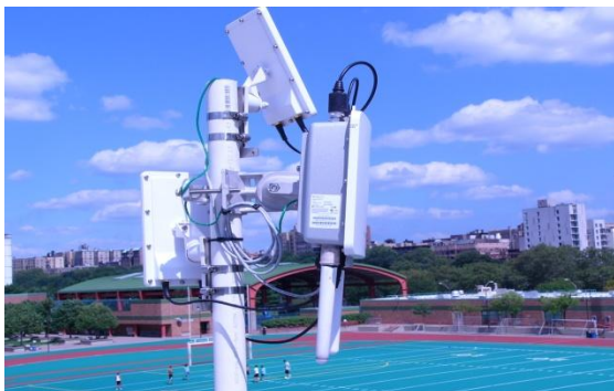
DDP Wi-Fi Radio at Riverbank State Park
